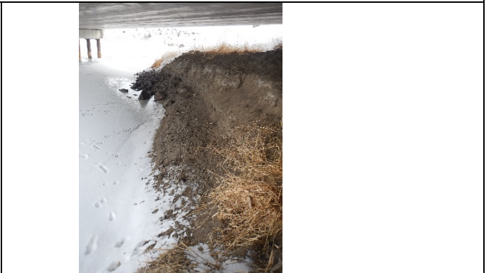
Photo 6. 19910: Inside structure, west-side. During high flow no pathway is available.
