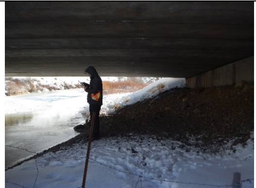
Photo 18. 19916: Inside structure, west-side. Slope could be graded and leveled to create dry, rip rap free passage.
