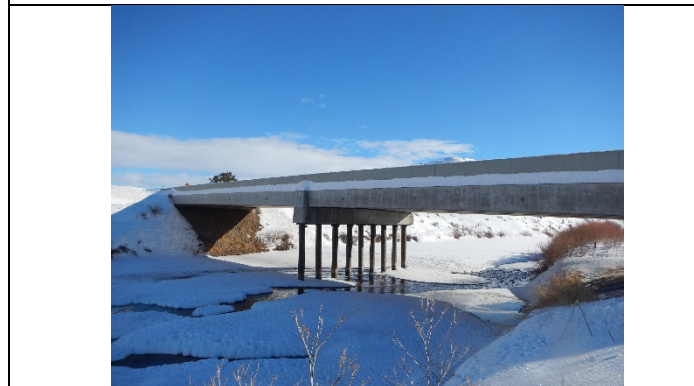
Photo 9. 19910: Outflow, east side of structure has steep embankment limiting function as passage
