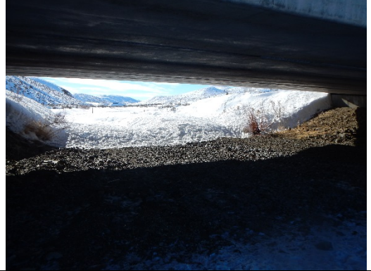
Photo 18. 19916: Inside structure, west-side. Slope could be graded and leveled to create dry, rip rap free passage.
