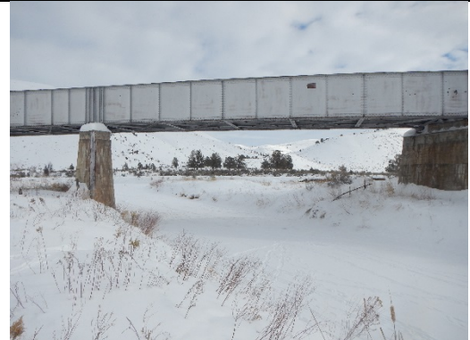
Photo 2. 19908: Outlet side facing railroad bridge. Note wire strand fences block wildlife passage.
