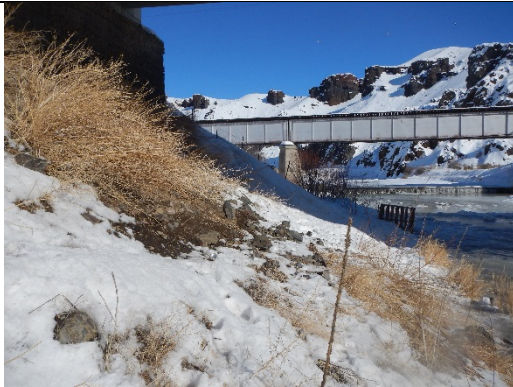
Photo 15. 19915: West-side pathway inside structure. Note: steepness of bank and fence interrupting pathway
