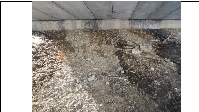
Photo 10. 19910: Inside structure, west-side. Slope could be graded and leveled to create dry, ice-free passage.
