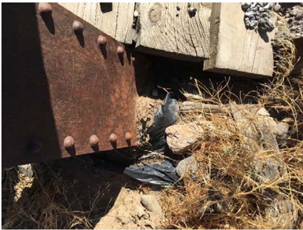
Photo 13. Buried End Post (Southwest Corner)
