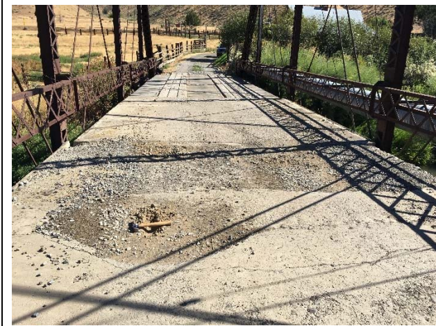
Photo 5. Deterioration of Concrete Deck
