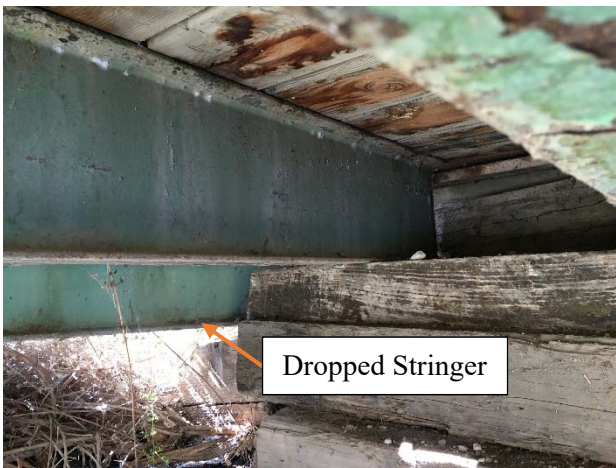
Photo 15. Dropped Stringer at Southeast Corner
